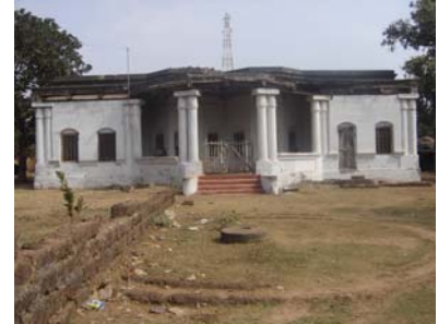
Fig. 11.27: Under utilized colonial bungalow in need of rehabilitation
